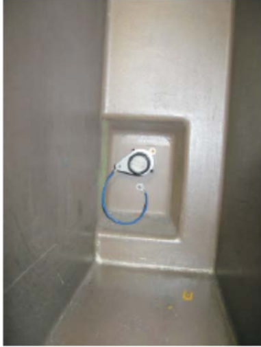
Shorting Cap Installed
